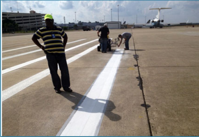
Workers install paint markings on the FAA ramp of Atlantic City International Airport. (Photo: FAA)
